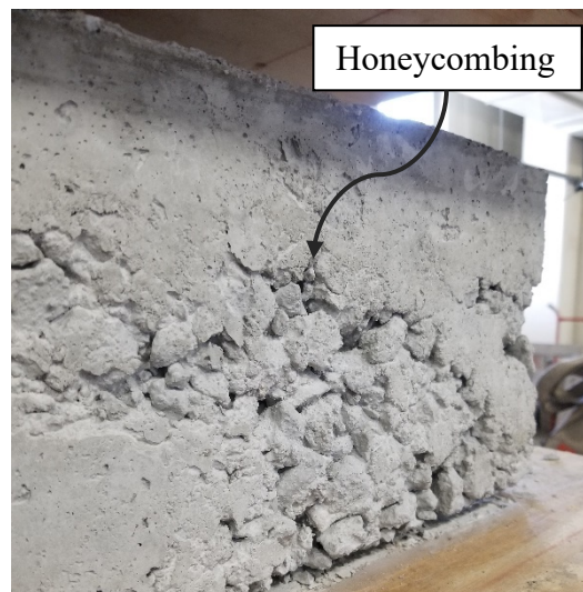
Figure 2-3: Honeycombing in a Concrete Slab
