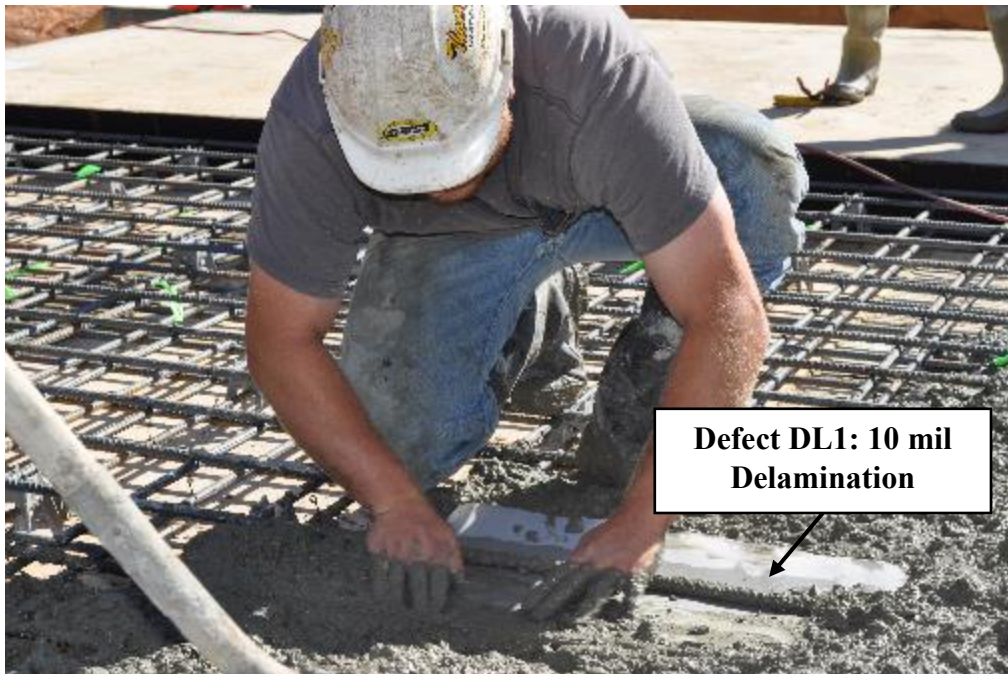
Figure 5-5: Plastic Sheetting Delamination Simulation in Test Bridge
