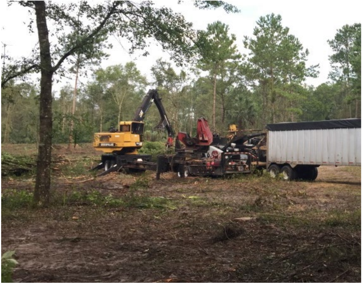
Figure 18: CAT 559D trailer mounted loader from operation B feeding a Bandit 3590 whole-tree chipper on the second landing.
