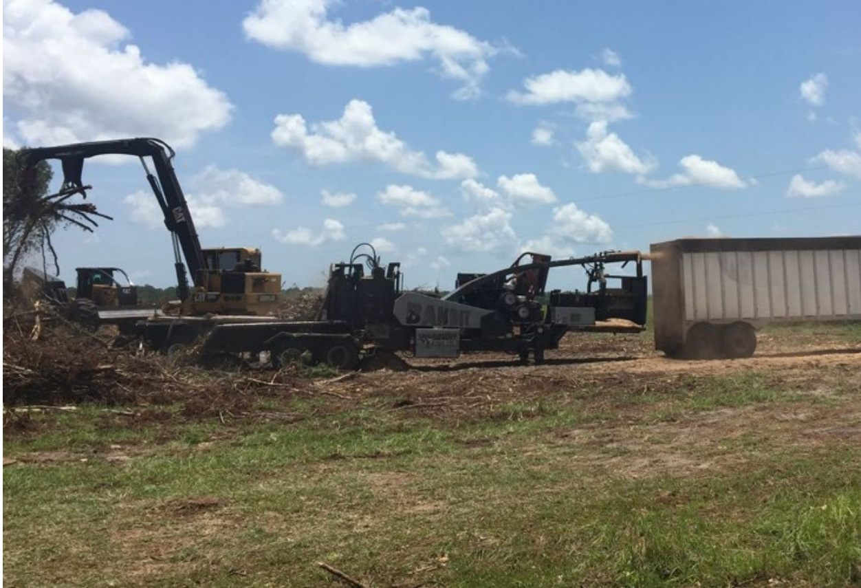
Figure 19: Bandit 3590 whole-tree chipper from operation B being fed by CAT 559D trailer mounted loader and blowing chips into chip trailer on the first landing.
