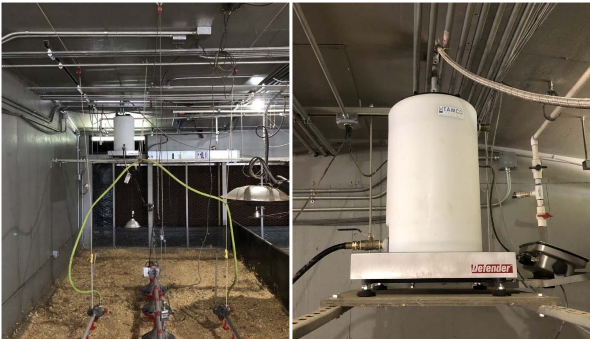
Figure 2.1. (left) Two water lines were installed either side of auger feed lines. (right) Water tanks with a capacity of 37.8 L were installed 1.4 m above the pen floor and supplied water to two drinker lines.
