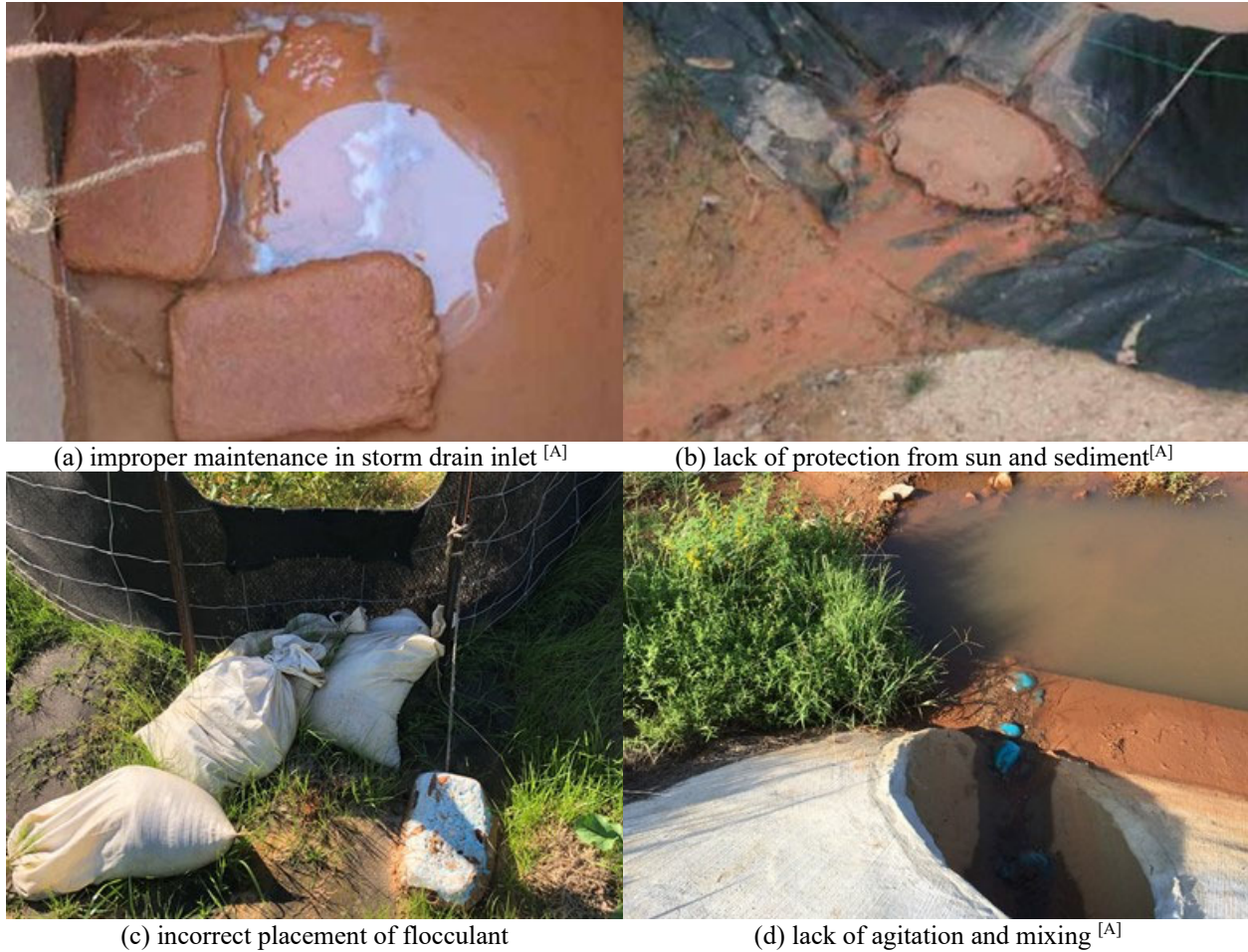
Figure 4 Poorly implemented flocculant applications.
