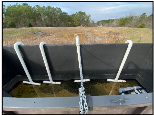
(b) PVC Pipe Water Delivery System
