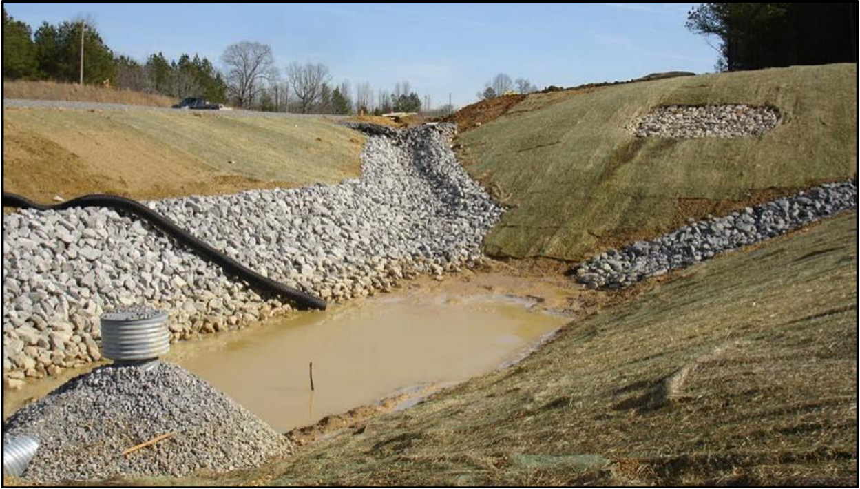
Figure 11 Riser Structure in ALDOT Sediment Basin (Perez, 2016).
