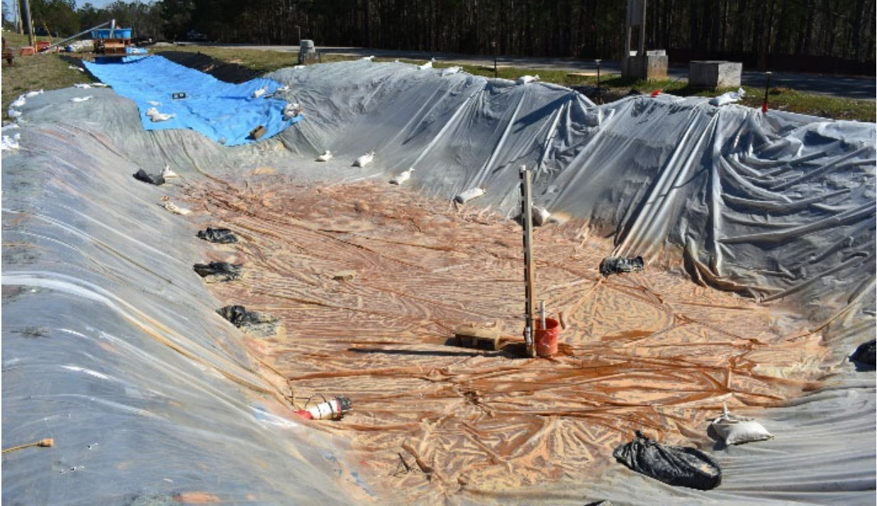
(a) Empty basin pre-test
