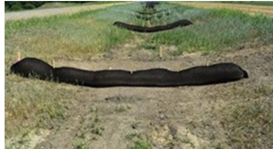
(b) W-S field installation
