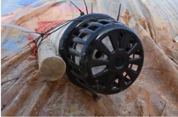
(a) basin side of dewatering pipe
