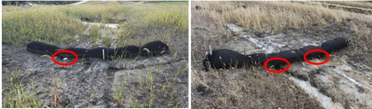
(a) undercutting upstream
