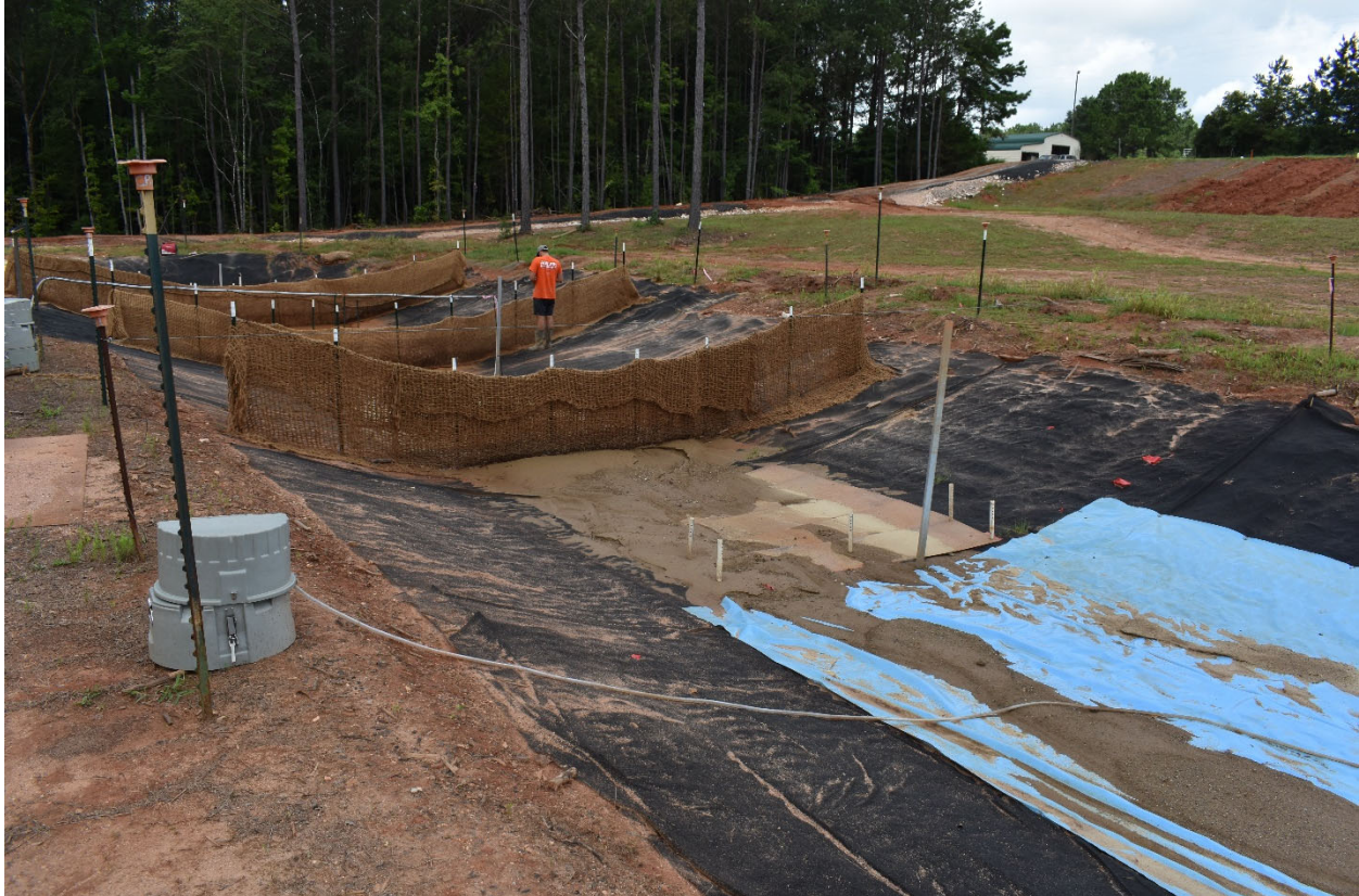
Figure 4.26. In-channel sedimentation due to coir baffle installation.
