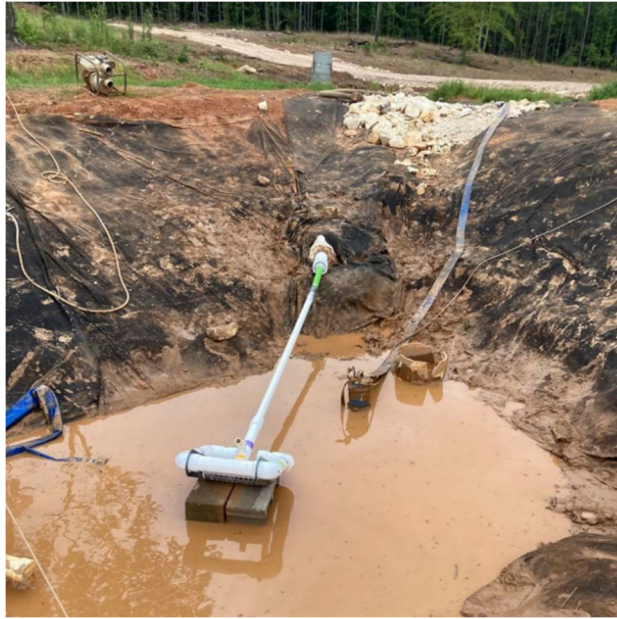
(a) skimmer resting on cinder blocks
