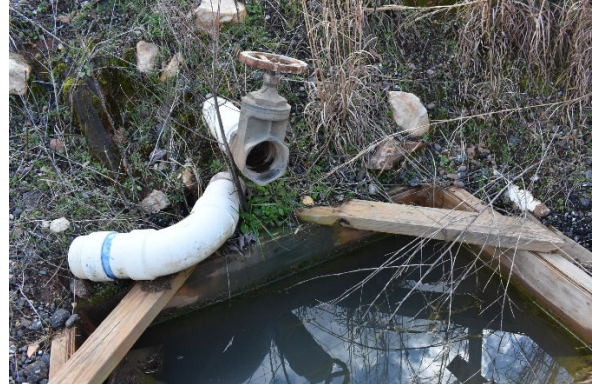
(b) downstream dewatering pipe
