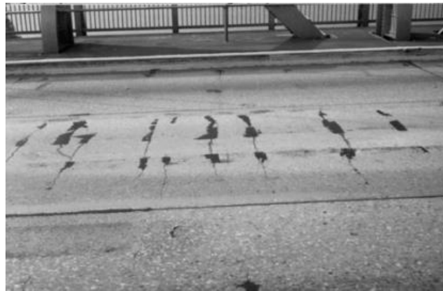
Figure 1.6: Typical deck transverse cracking (Adapted from Russell, 2004)
