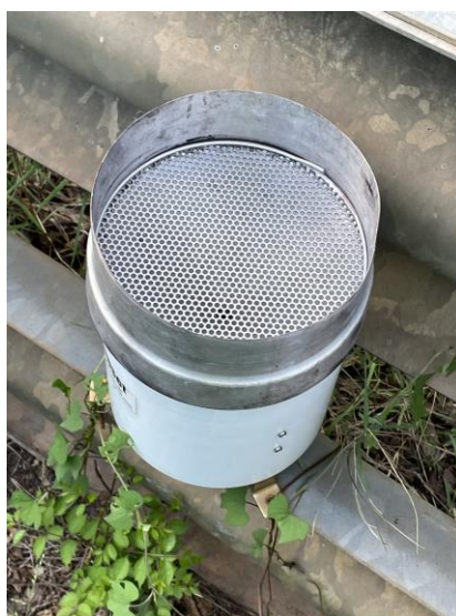
Figure 28. Rain gage deployed in Bridge BrM No 015002
